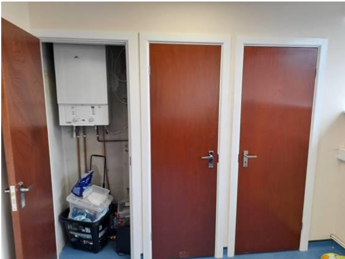
Above We can heat the entire parish hall with this single combi-boiler. It's a snug fit inside this narrow cupboard, itself built as part of a bespoke storage area in our new meeting room. More storage resides behind the other two doors.
