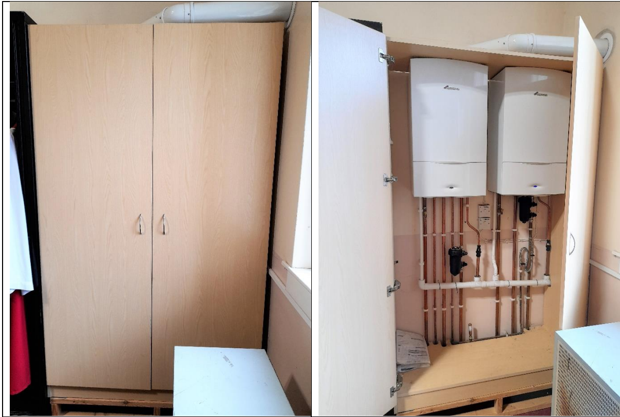
Above We can easily hide the two new Church boilers easily inside a standard wardrobe.
